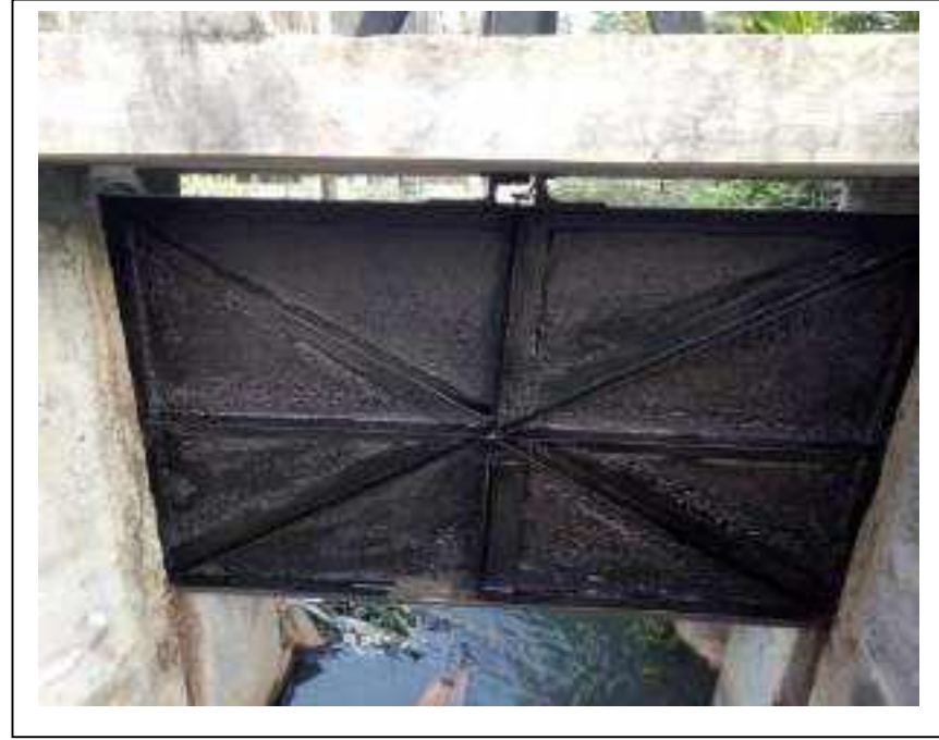
HALISAHAR DRAIN LOCKGATE
